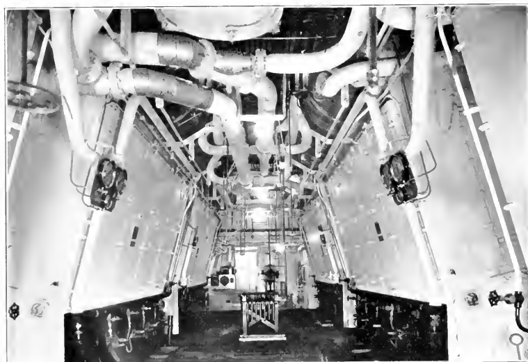
One of the firerooms of the Steamship President Coolidge, showing the very neat installation of steam piping and featuring the furnace fronts of four of the twelve Babcock & Wilcox interdeck, superheat type, marine, water-tube boilers. The high pressure steam pipes are covered with 85 per cent. Magnesia and with Johns-Manville Super-Ex insulation material. Fuel oil for these boilers is measured by Empire oil meters.
